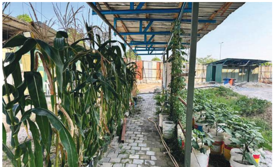
Enhancing on-site biodiversity through worker-led planting initiatives that integrate greenery into the construction environment.
